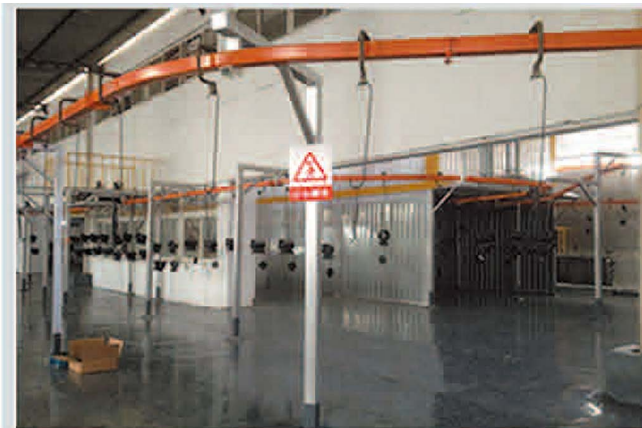
Automatic spraying production line
